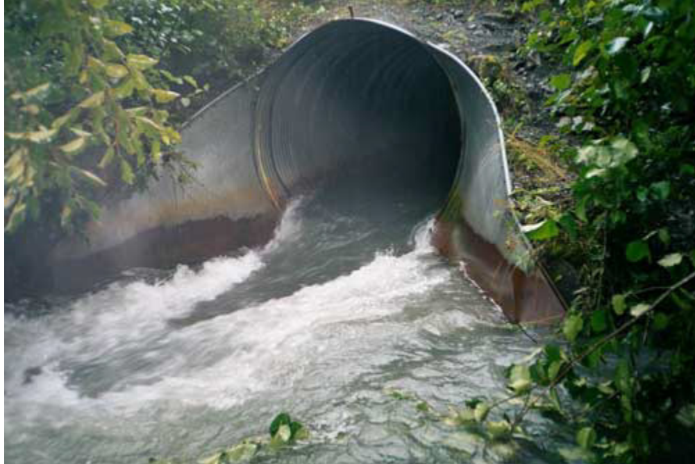
This culvert is undersized and the water velocity is too fast.
